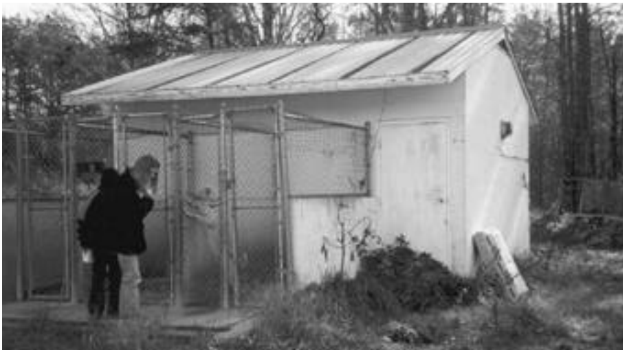
Compliance issues ranged from minor improvements to the need to replace entire facilities.
